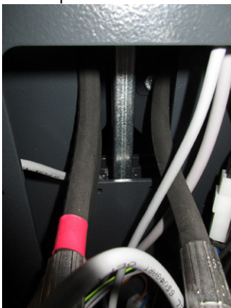
Location and orientation of the hydraulic hoses and cables.
